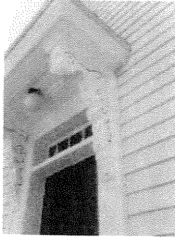
Reading 225- Exterior, A Side Decorative Molding
