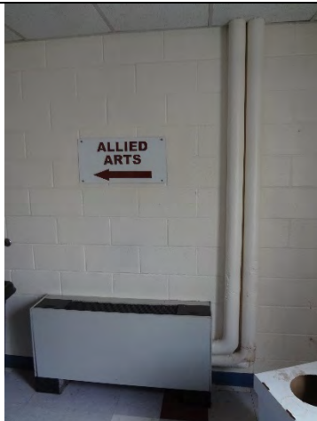
Figure H5: Clean & Repair Cabinet Unit Heaters (M)
