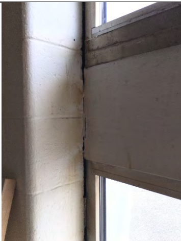
Figure A113: Interior Finish Issues at Precast Wall System (H)
