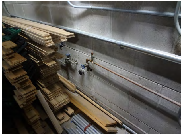
Figure P12: Abandoned Sink Piping (H)
