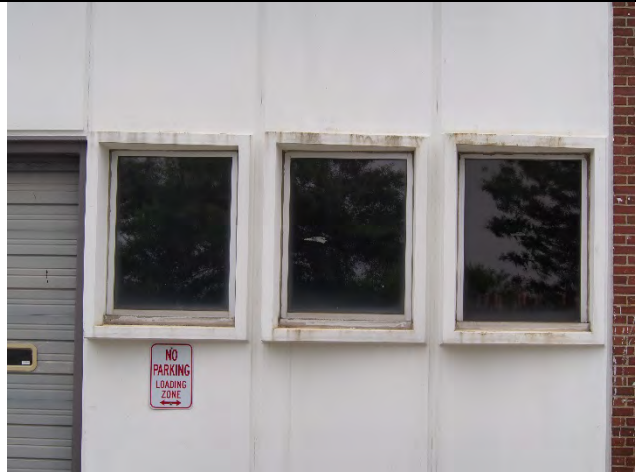
Figure A116: Precast Window System (H)
