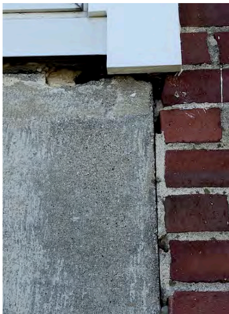
a. Open Mortar joints
