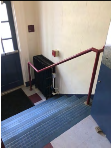
Figure A61: Stair Handrail – Life Safety Compliance Issues (EM)
