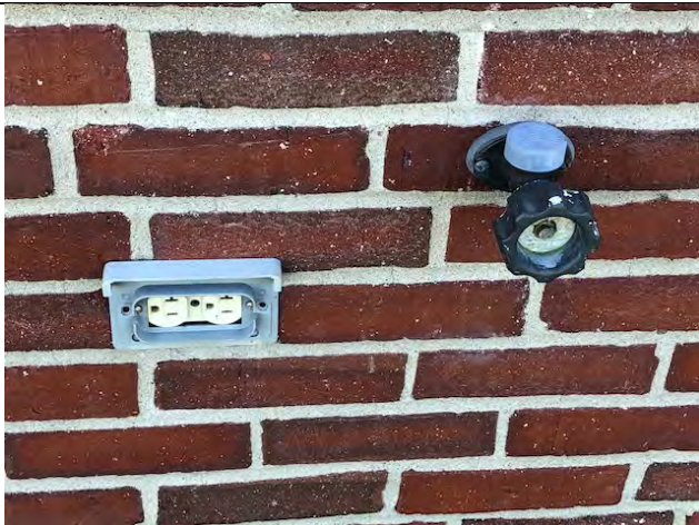
Figure A35: Exposed Outlet (non-GFCI) (EM)
