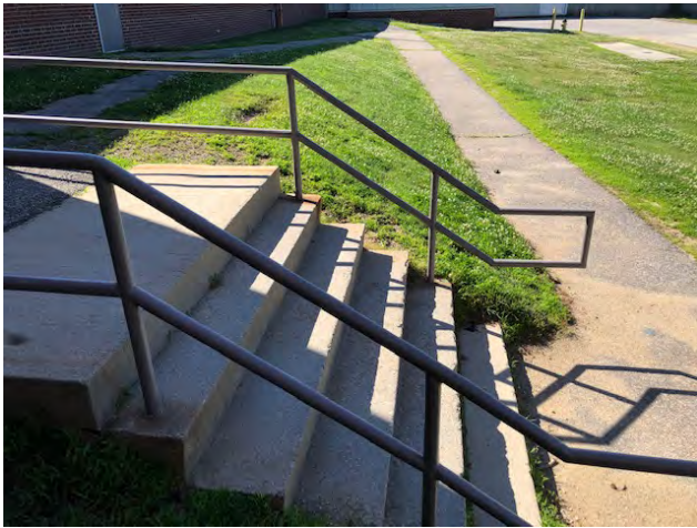
Figure A37: Non-Compliant Steps (EM)
