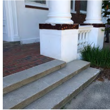
Figure A44: 1934 Building – Rusted Column Bases (EM)
