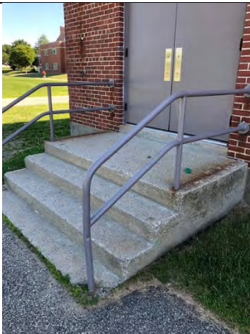
Figure A29: Non-Compliant Egress Door (EM)
