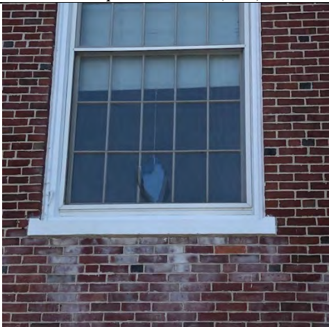
Figure A41: 1934 Building – Exterior Wall Water Staining (EM)
