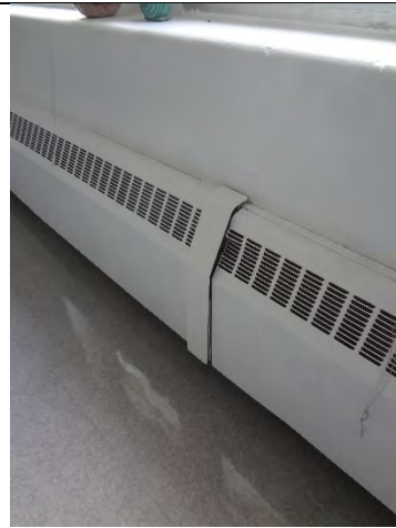
Figure H4: Fintube Radiator Covers (H)
