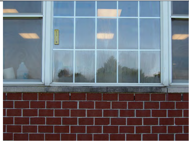
Figure A8: Failing Precast Window Sill (EM)
