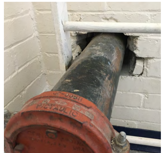
Penetration through stair wall not sealed.
