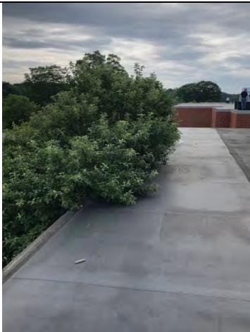
Figure A69: Vegetative Growth over EPDM Roofing (EM)
