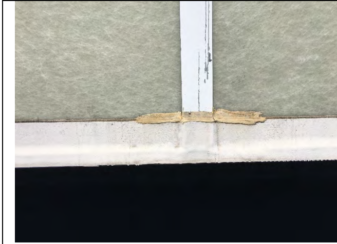
Figure A19: Skylight Conditions Issues (EM)
