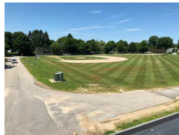
Figure A64: Site Issues at Middle School Ballfield (EM)
