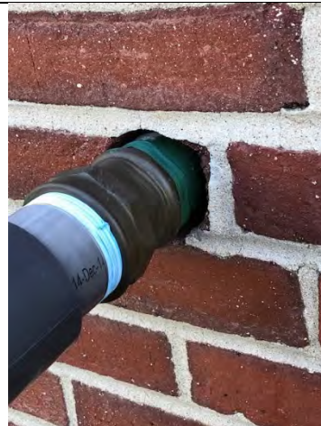
Figure A36: Unsealed Wall Penetration (EM)
