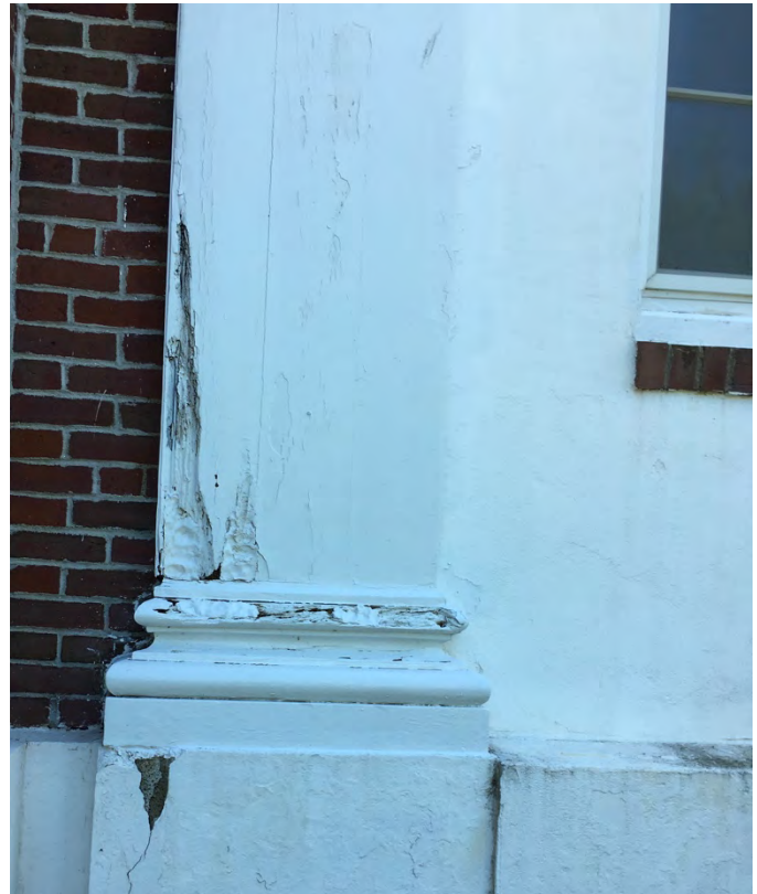
Spalling concrete at foundation and wood rot
