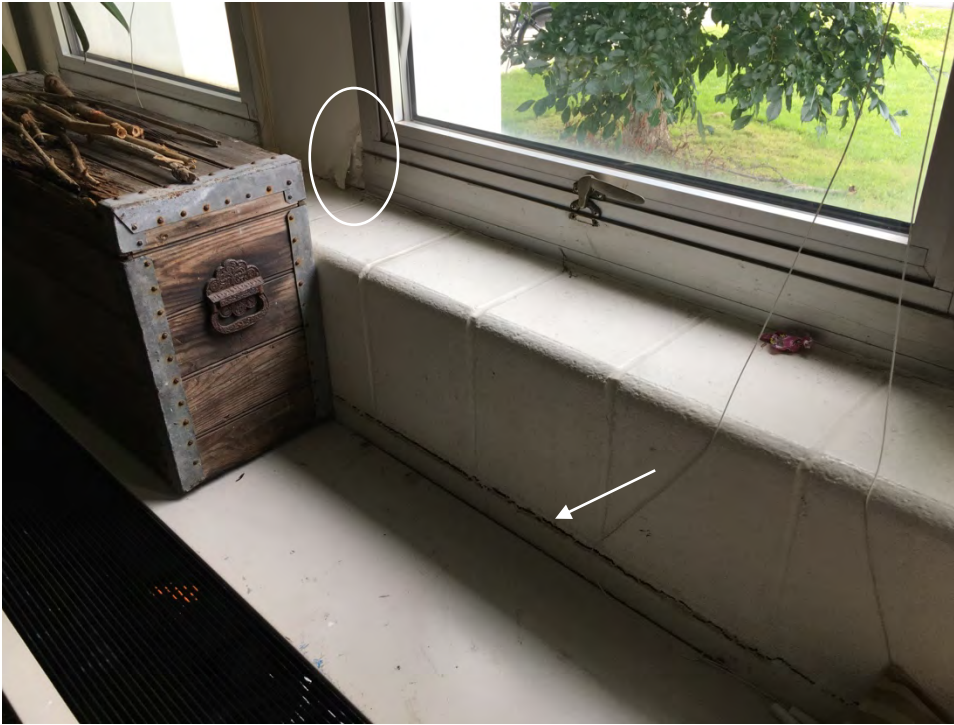
Drywall peeling from moisture infiltration / condensation and CMU cracking.
