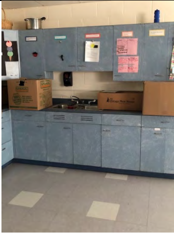
Figure A55: Life Skills – Non-ADA Compliant Sink (EM)
