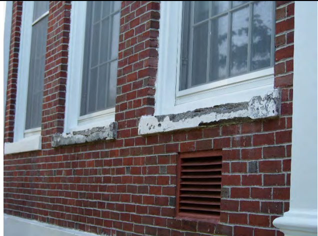
Figure A2: 1934 Building – Cast Stone Sill Damage (EM)
