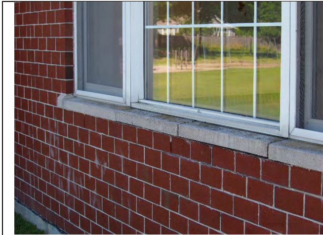
Figure A7: Failing Precast Window Sill (EM)
