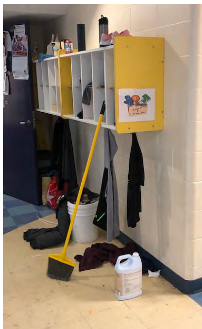
Lobby C120 Cubbies protrude beyond ADA limits
