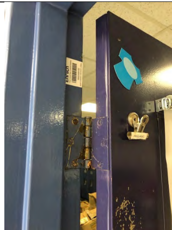
Figure A82: Classroom Door Rating Labeling (EM)
