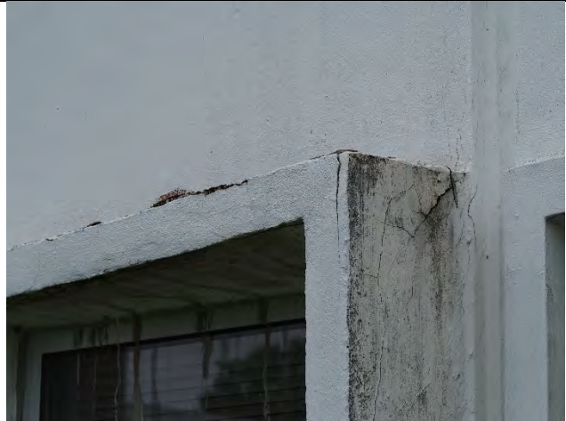
Figure A118: Moisture Issues at Precast Window System (H)
