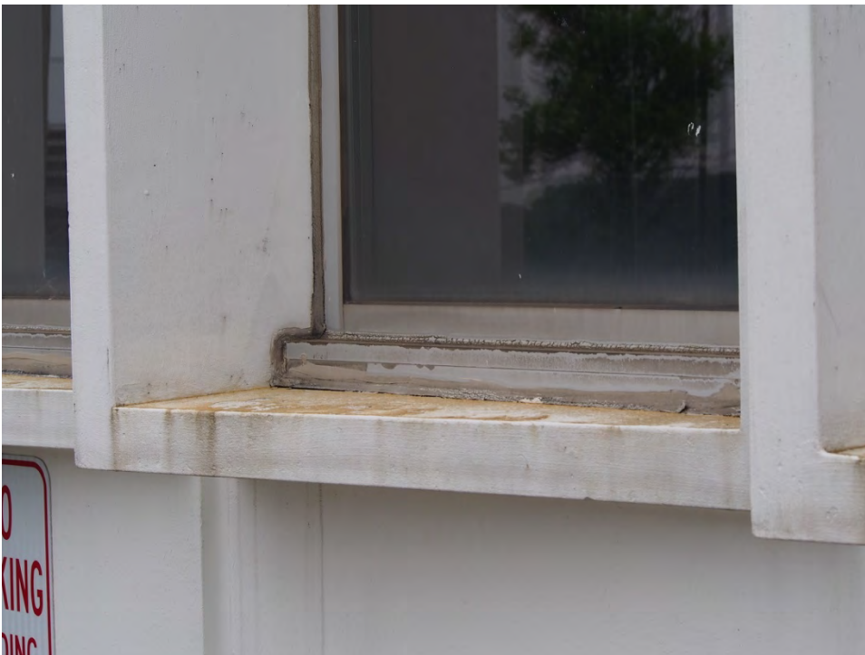
Non-thermally broken aluminum frames set into precast concrete panel are a vessel for condensation to form on the interior surfaces.
