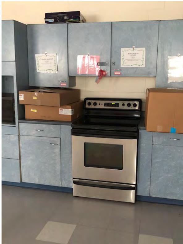
Range lacks an NFPA compliant exhaust and suppression hood
