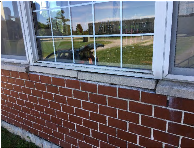
Figure A3: Failing Precast Window Sill (EM)
