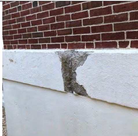
Figure A42: 1934 Building – Spalled Concrete at Foundation (EM)
