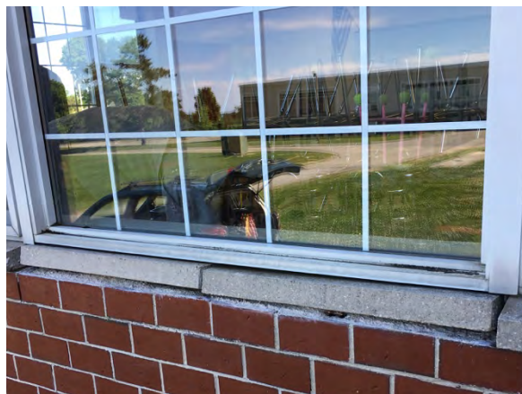
Dislodged precast window sills
