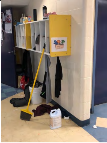
Figure A85: Non-ADA Compliant Wall Cubbies (EM)
