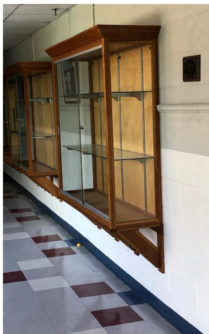
Corridor D117 Display cases protrude beyond ADA limits
