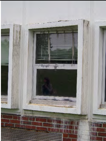
Figure A117: Moisture Issues at Precast Window System (H)
