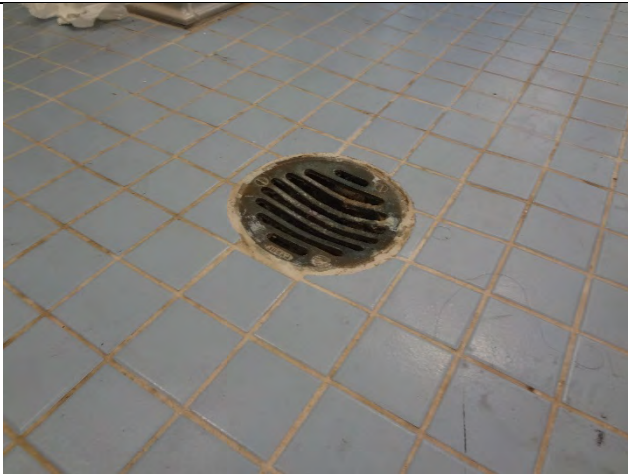
Figure P3: Damaged Drain Gate (M)
