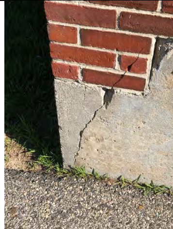
Figure A28: Crack at Concrete Foundation and Brick (EM)
