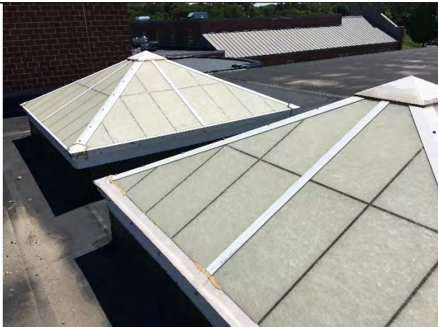
Figure A17: Skylight Conditions Issues (EM)
