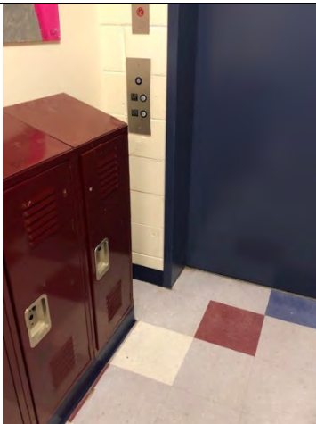
Figure A63: Non-ADA Compliant Elevator Lobby (EM)
