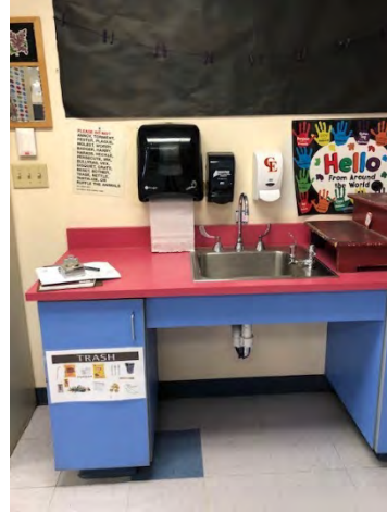
Figure A74: Non-ADA Compliant Sink (EM)
