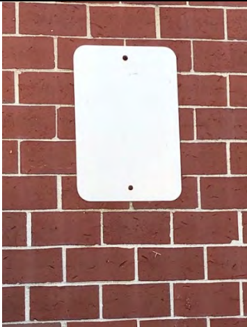
Figure A33: Sun Damaged Sign (EM)
