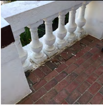
Figure A45: 1934 Building – Cracked Brick Paving (EM)
