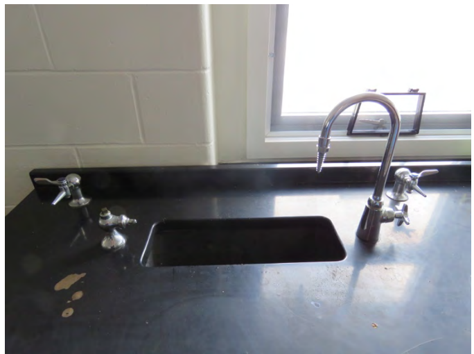
Lab sink is too small.
