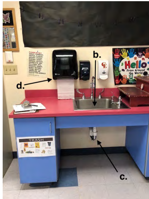
Example non-ADA compliant classroom sink, E109
