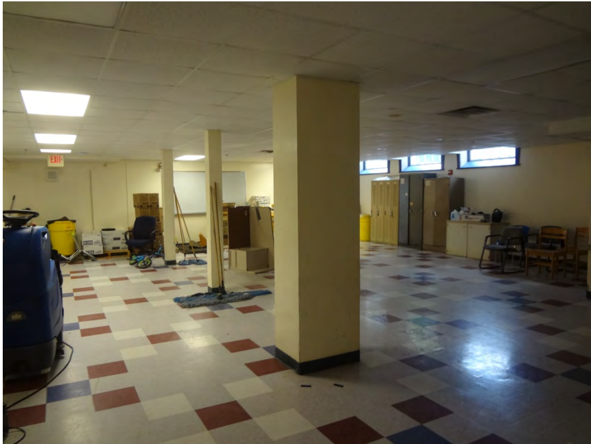
Area to left of columns must be a defined egress corridor with a UL partition.
