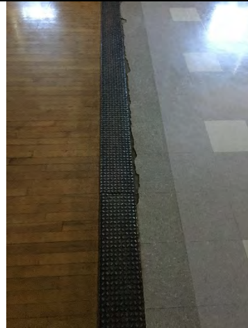
Figure A14: Flooring Damage at Band Room (EM)
