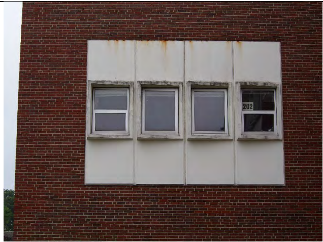
Figure A122: Rust Stains at Precast Window System (H)
