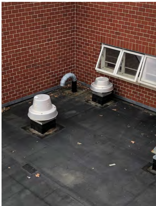
Operable window unit within ten feet of exhaust hood
