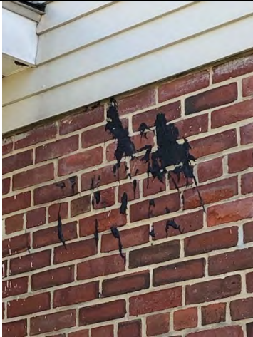
Figure A27: Exterior Wall Mastic Staining (EM)
