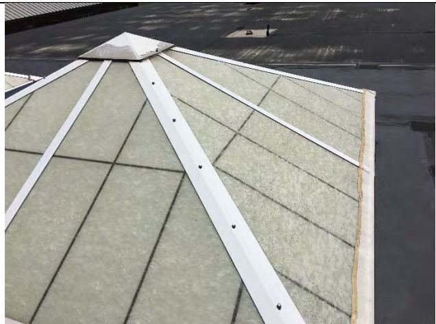
Figure A18: Skylight Conditions Issues (EM)
