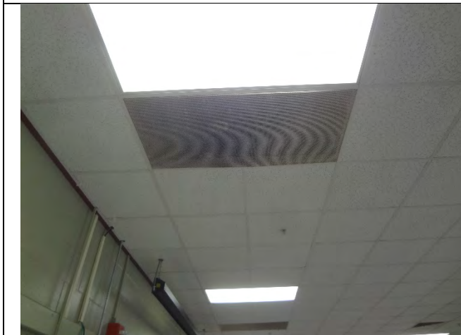
Figure H11: Sagging Return Grilles (H)
