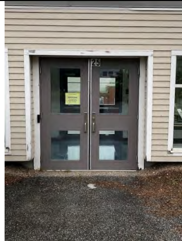
Figure A104: Door #25 (EM)
