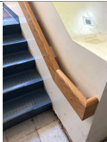
Figure A66: Stair Handrail – Life Safety Compliance Issues (EM)
