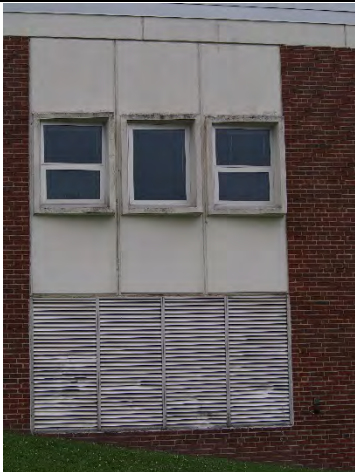
Figure A123: Precast Window System with Abandoned and Damaged Wall Louver (H)
