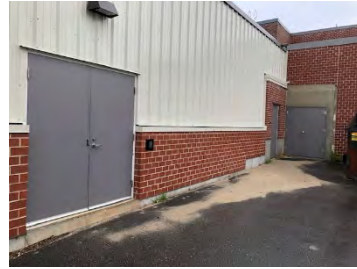
Figure A110: Un-numbered doors at Storage/Boiler Room (EM)
