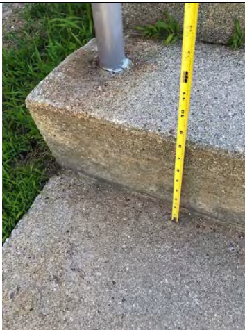
Figure A39: Stair Riser Height – Life Safety Compliance Issue (EM)
