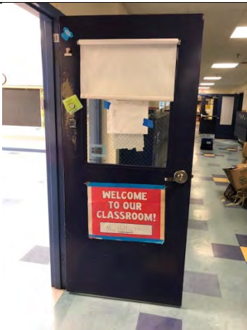
Figure A81: Classroom Door without Closer – Life Safety (EM)
