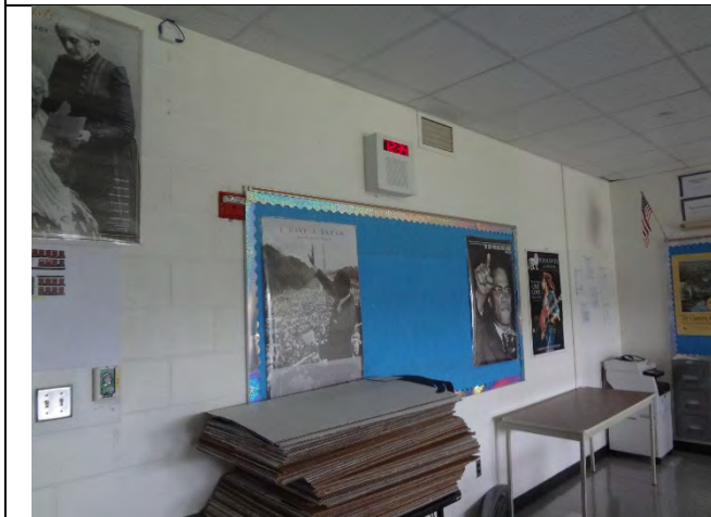
Figure H9: Broken Temperature Sensor (H)
