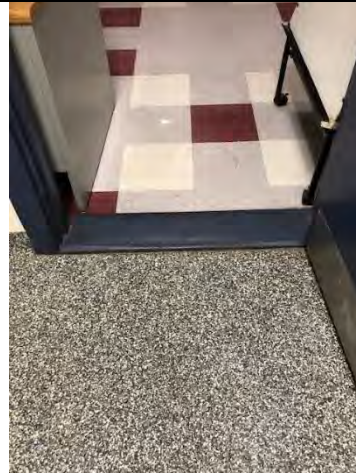
Figure A62: Non-ADA Compliant Door Threshold (EM)
