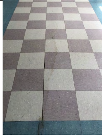
Figure A50: Buckling at Floor Ramp (EM)
