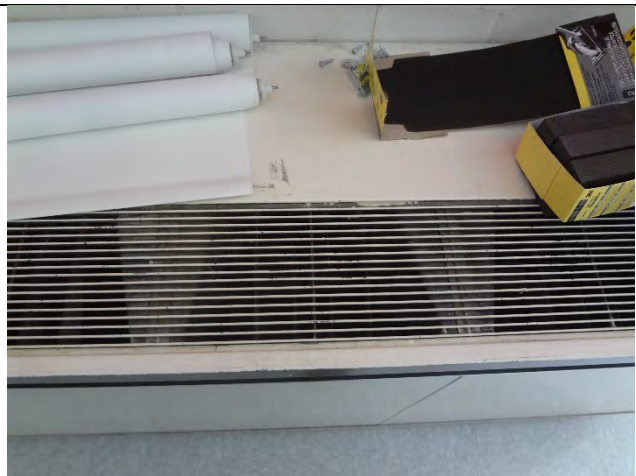
Figure H10: Clean Cabinet Unit Heater Interior (H)
