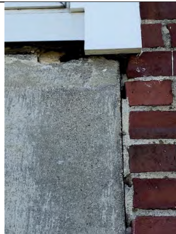
Figure A30: Missing Mortar at Brick/Concrete Intersection (EM)
