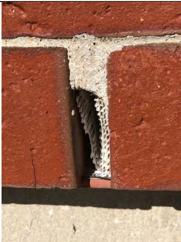
Figure A23: Degraded Masonry Weep (EM)
