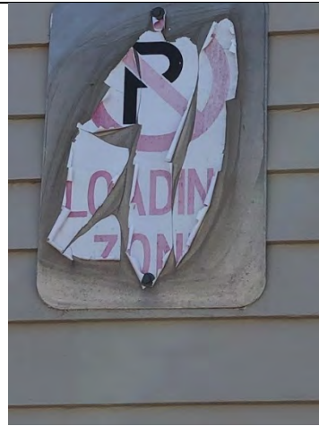
Figure A32: Damaged Sign (EM)
