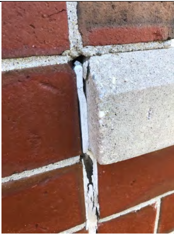
Figure A21: Sealant Issues at Window Sill (EM)
