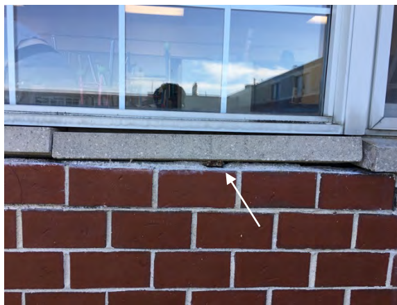
Embedded anchor no longer attached to backup
