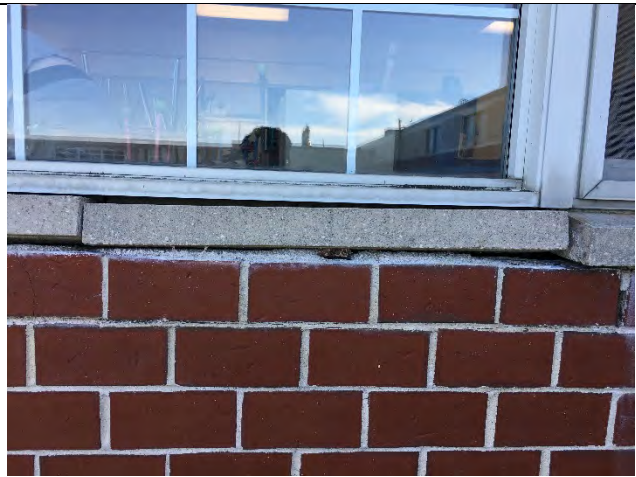
Figure A4: Failing Precast Window Sill (EM)
