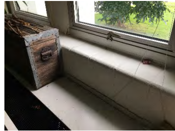
Figure A112: CMU Crack at Window Sill (H)
