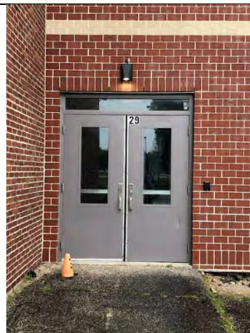
Figure A108: Door #29 (EM)
