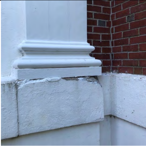
Figure A43: 1934 Building – Spalled Concrete at (EM) Foundation
