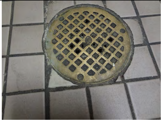
Figure P8: Plugged Drain Grate (H)
