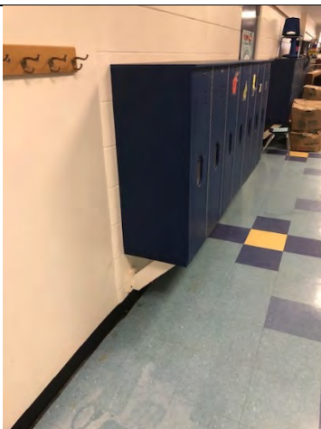
Figure A71: Non-ADA Compliant Wall Lockers (EM)
