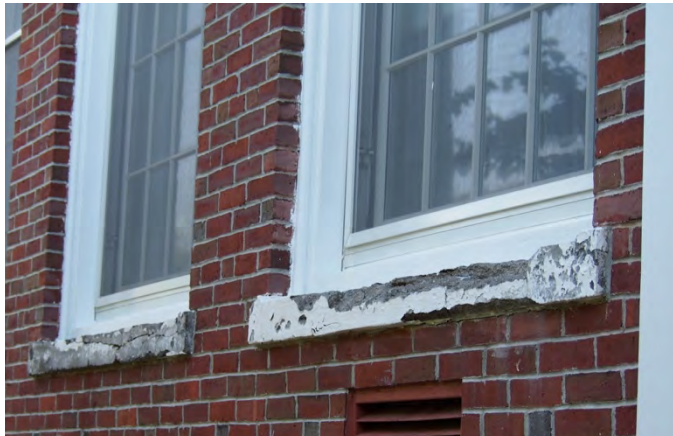
Deteriorating cast stone sills
