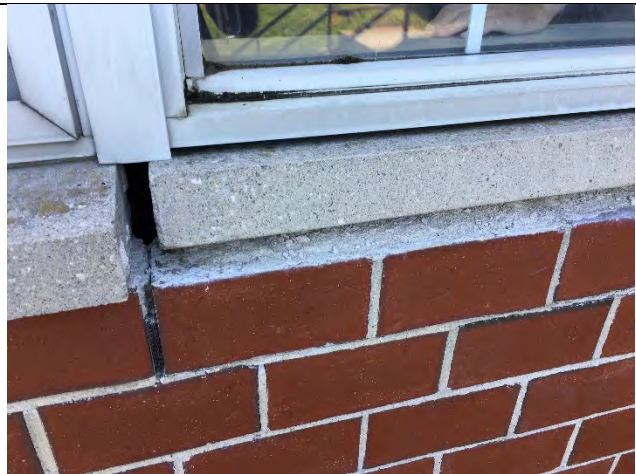
Figure A6: Failing Precast Window Sill (EM)
