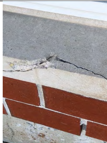
Figure A24: Crack at Precast Window Sill (EM)
