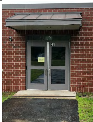
Figure A106: Door #27 (EM)
