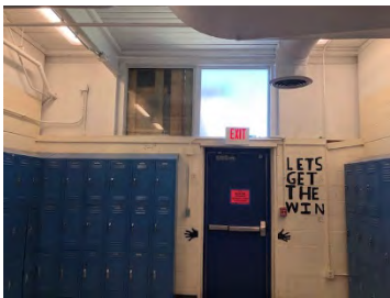
Figure A57: Locker Room Lacks Fire Separation from Boiler Room (EM)
