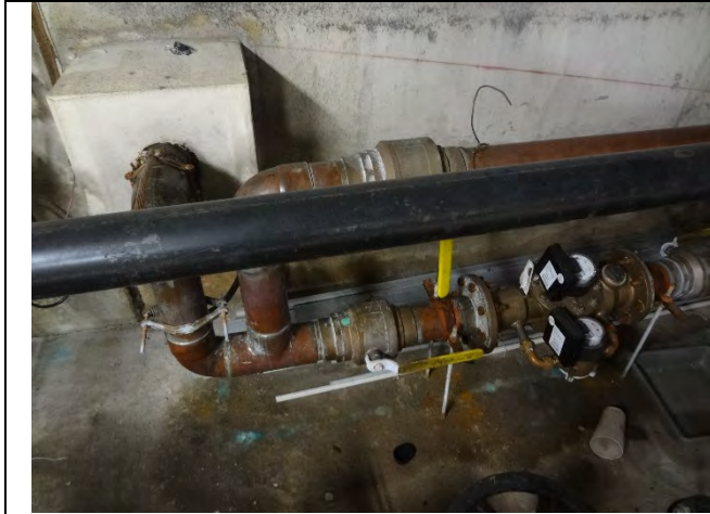
Figure P7: Water Meter bypass seal (H)
