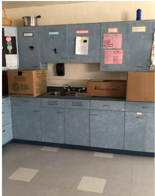
Sink is not ADA compliant
