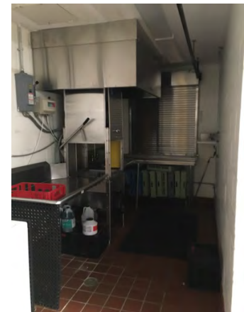
Dishwashing area is undersized.
