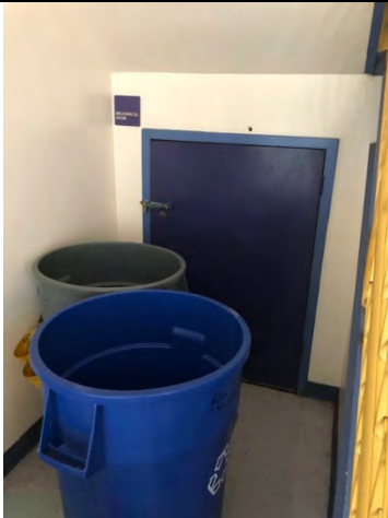
Figure A75: Storage below egress stair – Life Safety Compliance Issue (EM)
