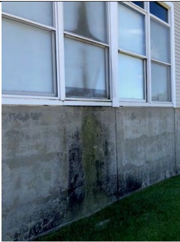
Figure A31: Water Staining and Biological Growth below Window (EM)
