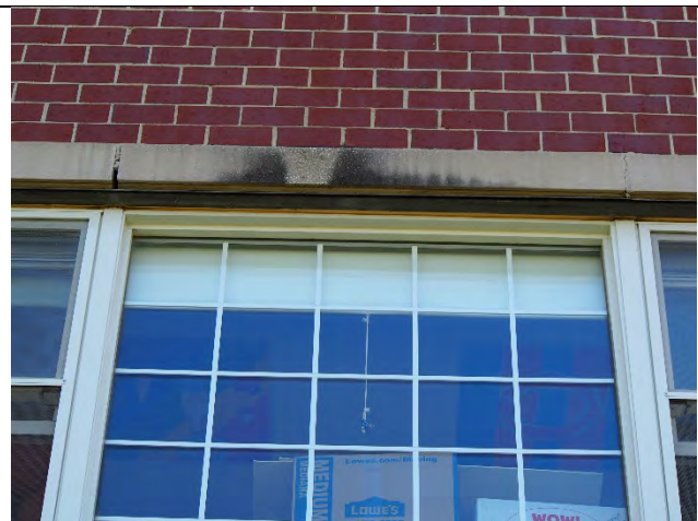
Figure A10: Failing Joints at Precast Window Head (EM)
