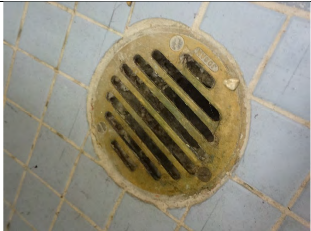
Figure P4: Plugged Shower Drains (M)
