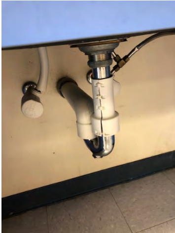
Figure A73: Non-ADA Compliant Sink Waste Trap (EM)
