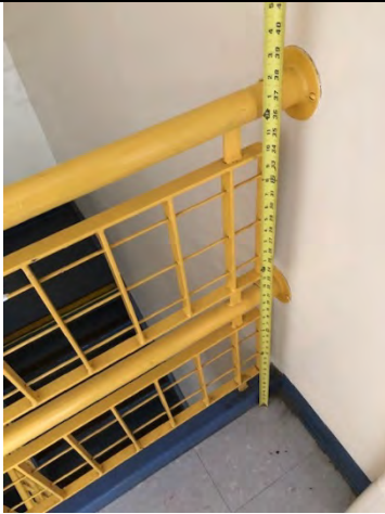
Figure A79: Stair Handrail – Life Safety Compliance Issues (EM)
