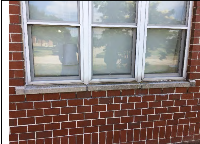
Figure A13: Water Spill and Masonry Damage at Window Sill (EM)
