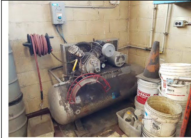
Figure H1: Metal Lab Air Compressor (H)
