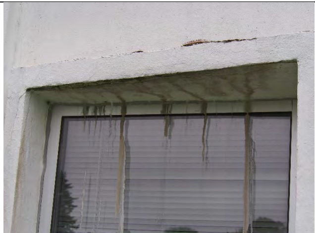
Figure A120: Moisture Issues at Precast Window System (H)
