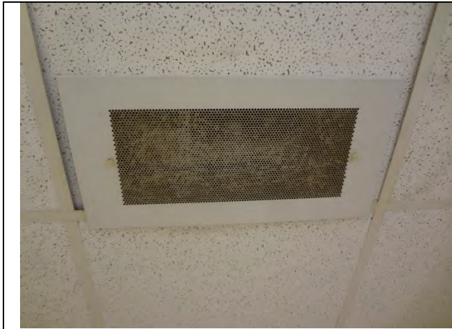
Figure H7: Clean and Support Fan (M)
