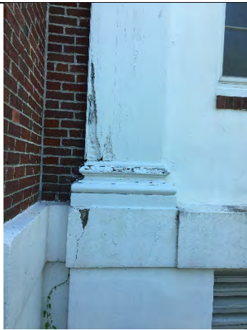
Figure A15: 1934 Building – Exterior Wood Rot (EM)
