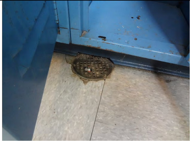
Figure P2: Plugged Drain Gate (M)
