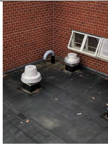
Figure A68: Window Located Adjacent to Exhaust (EM)
