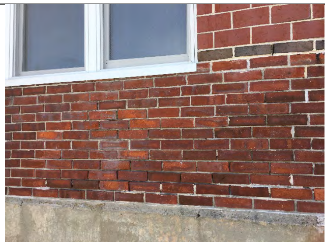
Figure A12: Brick Needs Repointing (EM)
