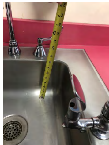
Figure A72: Non-ADA Compliant Sink (EM)
