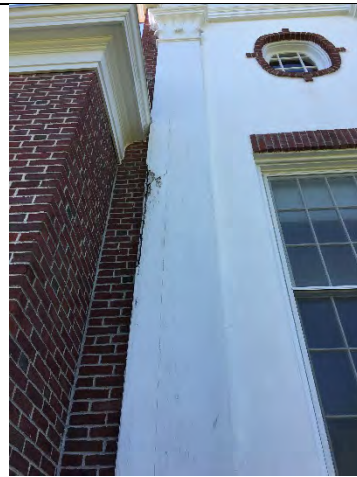
Figure A16: 1934 Building – Exterior Wood Rot (EM)
