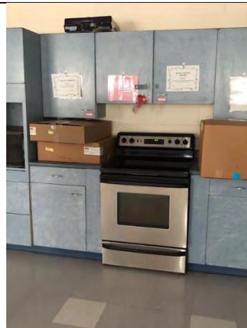
Figure A54: Life Skills – No Exhaust Hood at Range (EM)
