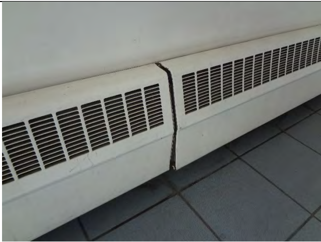
Figure H3: Fintube Radiator Covers (EM)
