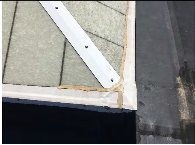
Figure A20: Skylight Conditions Issues (EM)
