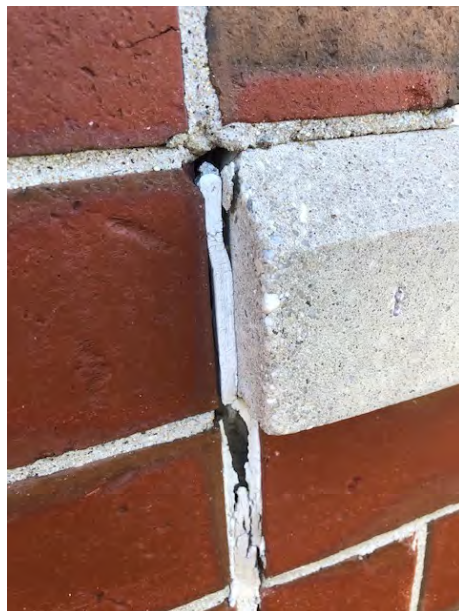
b. Failing soft joints
