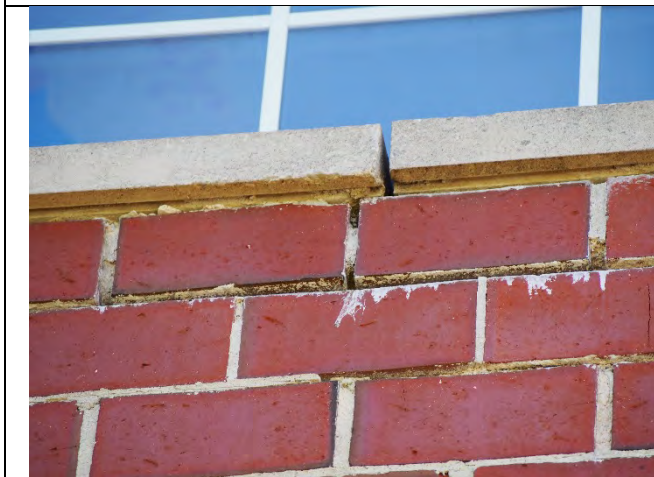
Figure A9: Failing Precast Window Sill (EM)
