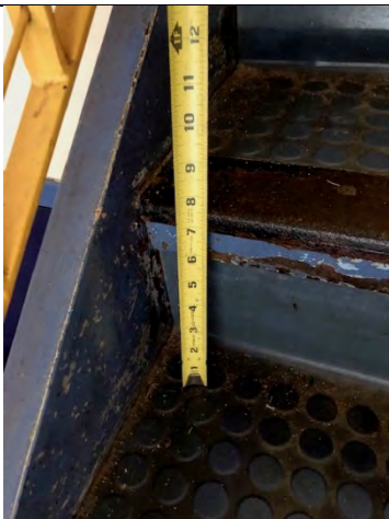
Figure A83: Stair Handrail – Life Safety Compliance Issues (EM)
