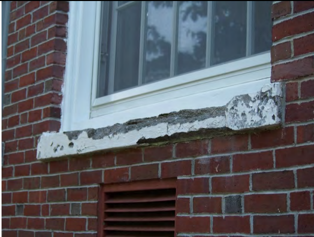
Figure A1: 1934 Building – Cast Stone Sill Damage (EM)
