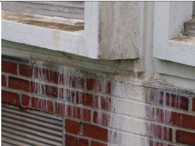
Figure A119: Moisture Issues at Precast Window System (H)
