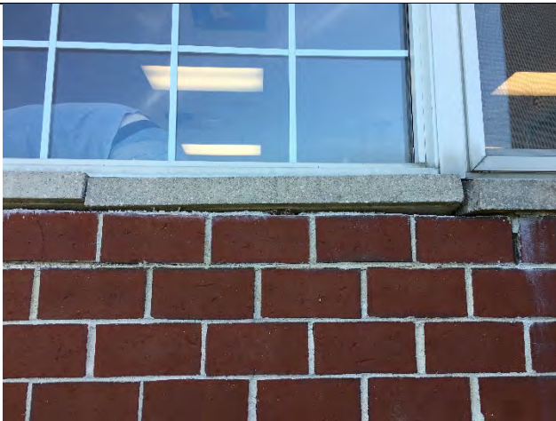
Figure A5: Failing Precast Window Sill (EM)
