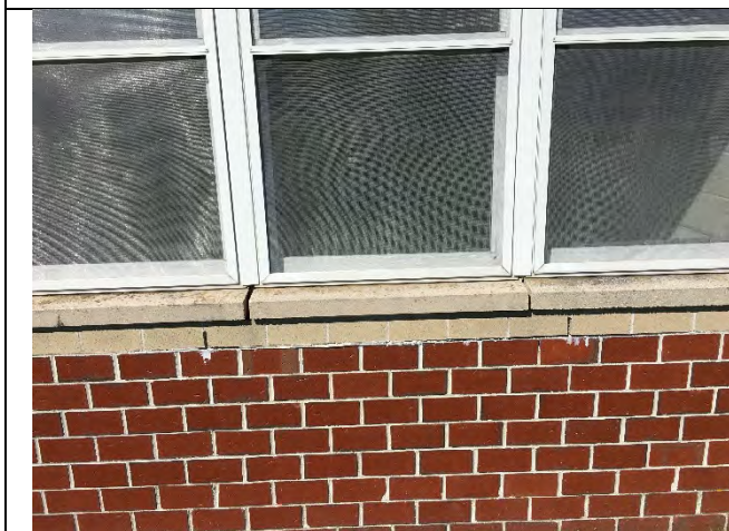
Figure A11: Failing Precast Window Sill (EM)
